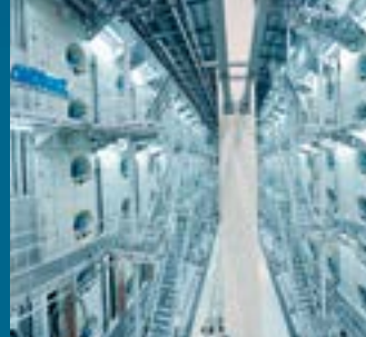
Pulp drying plant
